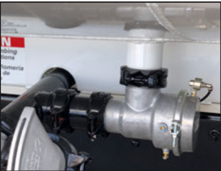
PRESSURE BYPASS VALVE Reduces water hammer by returning water to tank with pressure sensing air valve.
