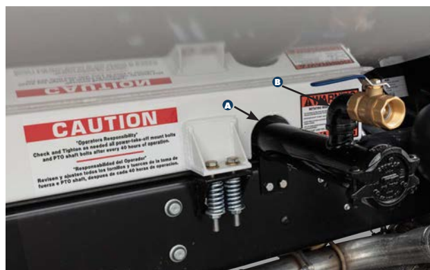
(A) Cut out arch in the tank runner for the manifold pipe mounted to the frame rail. (B) 1 1/2" brass jet valve mounted on passenger side of truck. Note the mounting bracket for the manifold pipe.
