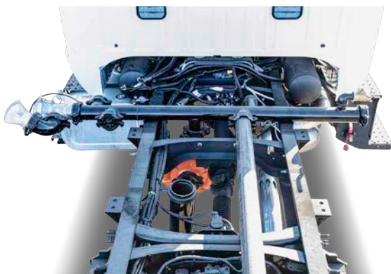
Top view of water pump mounted frame rail on driver side. Plumbed to manifold with rear supply pipe attached.
