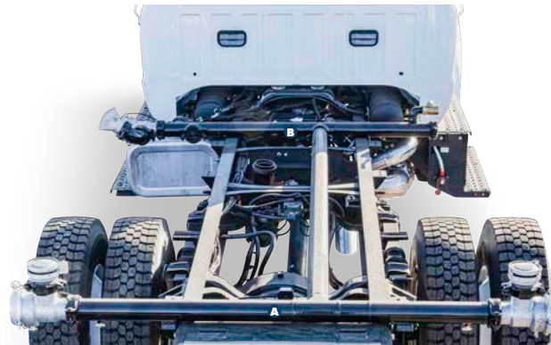
(A) The 3" rear spray bar tees into the supply line. (B) 3" manifold with grooved ends to be installed at a specified mid-ship location. The manifold pipe and rear bar pipe are mounted to the outside of the frame rail with bolt on brackets.
